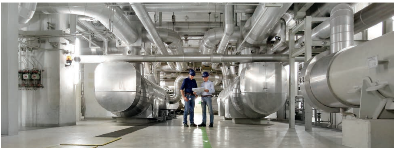
Employees at a preheater (Image: PreussenElektra; Photographer: Regine Rabanus)
