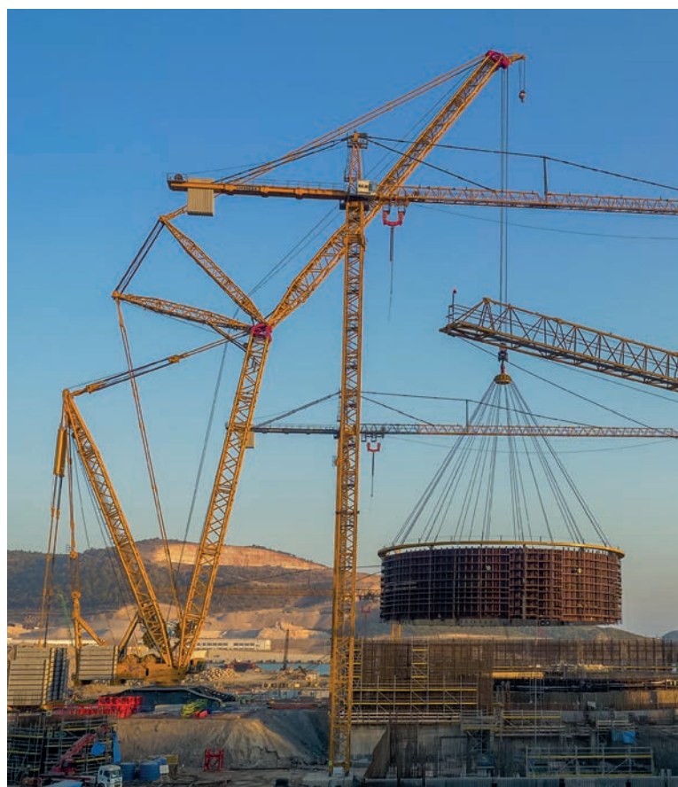
June 2020, Unit 1 reactor building inner containment second tier installation (Image: Akkuyu image bank, ROSATOM)
